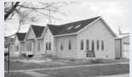
A new dentist office is underway for Ted B. Koester, DMD, PC. at the corner of First and Section Streets in Effingham. The practice welcomes new patients and uses the slogan..."Put an Extra Sparkle in Your Smile"
